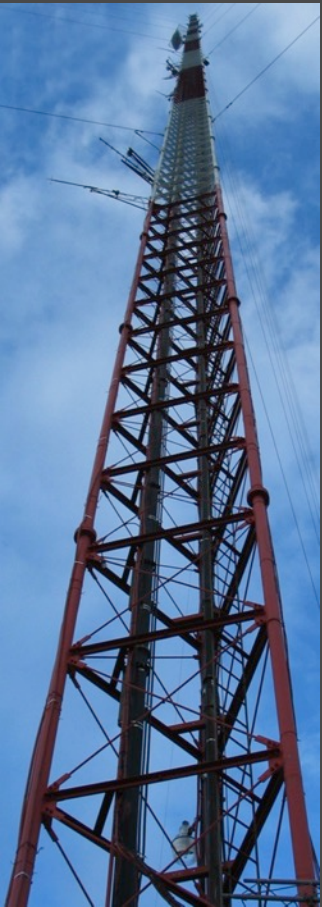
Communications towers ~100 m AGL
