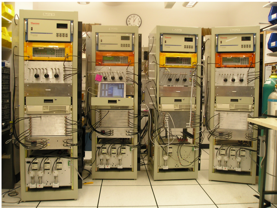
Figure 1: Four new tall towers measurement systems constructed at ESRL/GMD.
