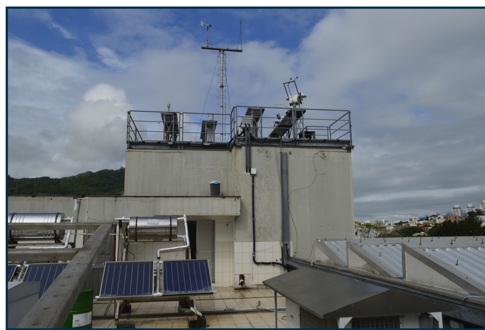
View of the solar water heating system and the BSRN Station.
