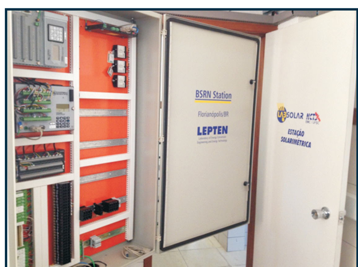
Indoor controls of the trackers and data collection
